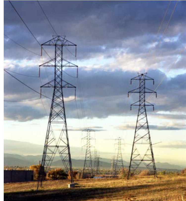
Photo by Werner Slocum, NREL 00001
