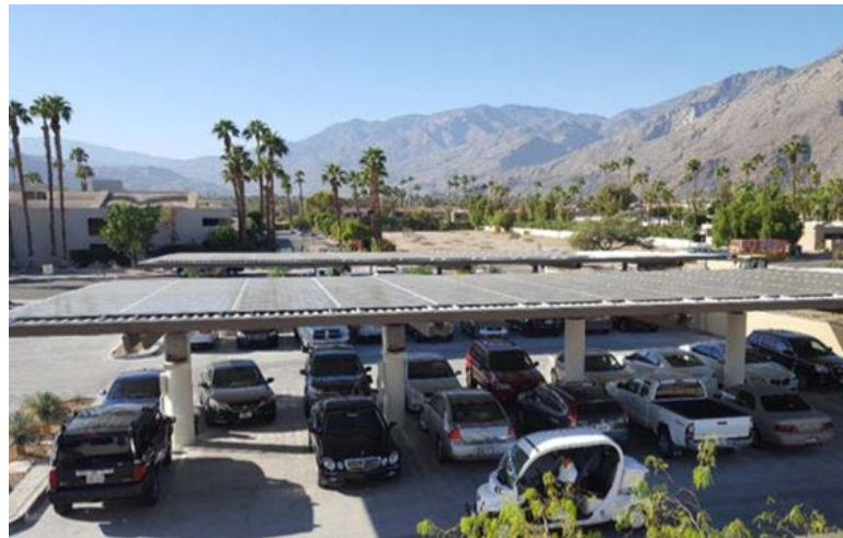
80-kW parking canopy solar system at Agua Caliente reduces Tribal office electricity cost from $22,000 to $200 annually.
