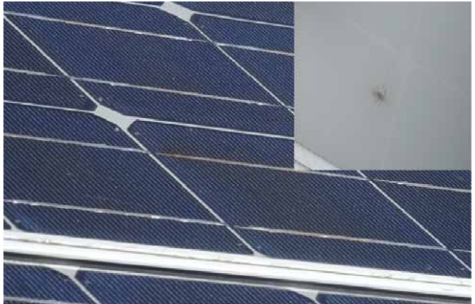
Figure 1. Solder bond failure leads to a hot spot visible (zoomed in top right) from the front and back. Photo by Dirk Jordan, NREL
