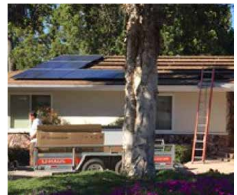
Figure 2. In California, shading of this PV system is the result of poor installation practices. Photo courtesy of homeowner.
