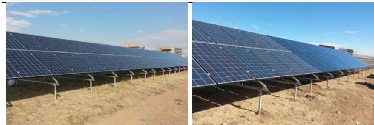
Figure 2. NREL PV Lifetime installations. Jinko Solar (left) and Trina Solar (right)
