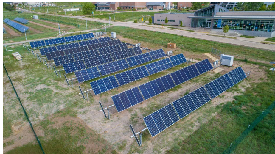
Figure 8. NREL 75-kW tracking PV system supporting PV Lifetime performance data
