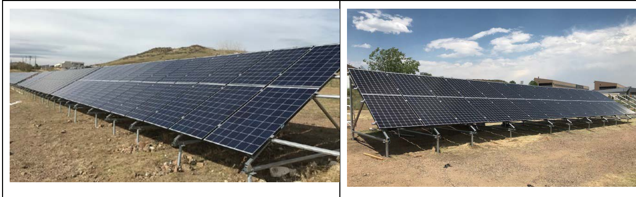
Figure 5. NREL PV Lifetime installations. QCells (left) and Panasonic (right)
