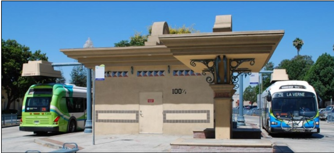
Figure 8. BEB charging station at the PTC
