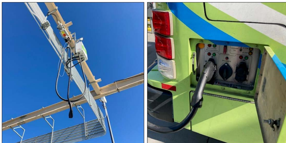
Figure 10. EVSE at Arcadia depot
