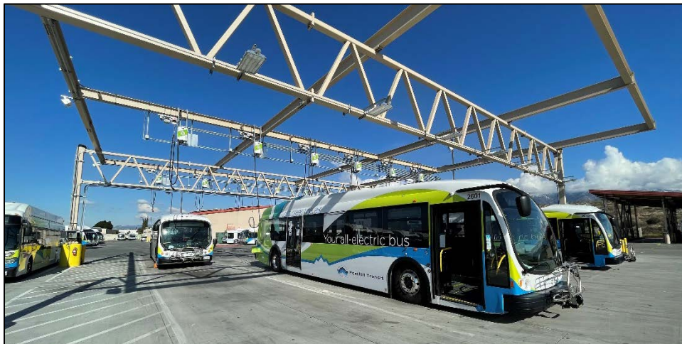
Figure 9. BEB charging structure at Arcadia depot
