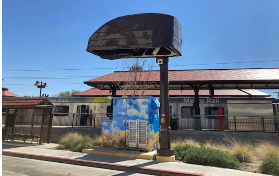
Figure 11. BEB charging station at AITC
