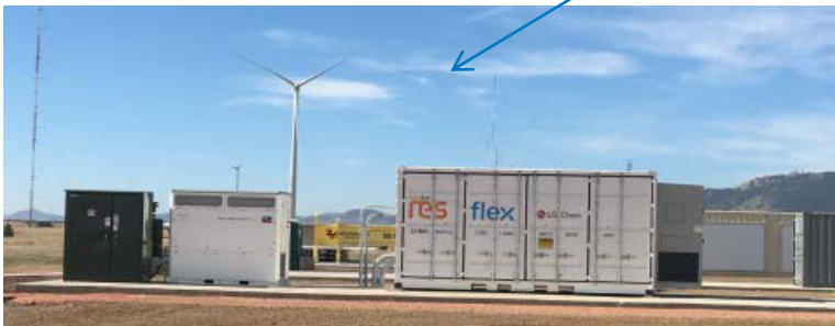
New: 1-MW/1-MWh battery
