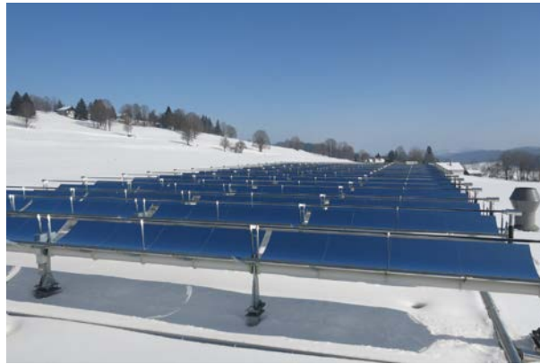
Figure 29. PolyTrough 1800 roof mounted solar field at the Saignelégier dairy processing plant in Switzerland (Minder 2013)
