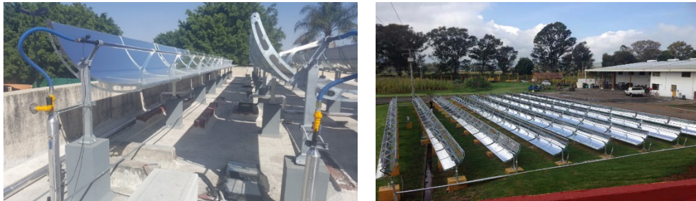
Figure 31. Roof-mounted Power Trough 110 solar field (left), and ground-mounted solar field (right). Photos from Inventive Power, credit: Inventive Power
