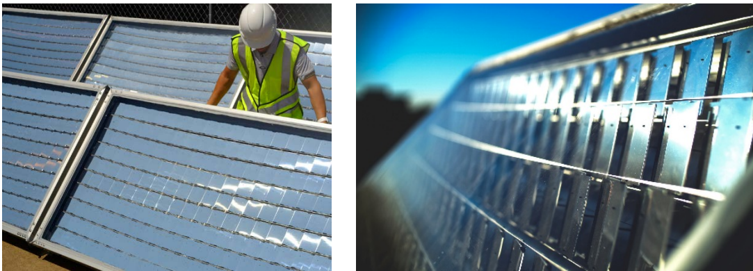
Figure 37. Skyven Technologies modular panels being installed (left), and close up (right). Photos from Skyven Technologies, credit: Skyven Technologies.
