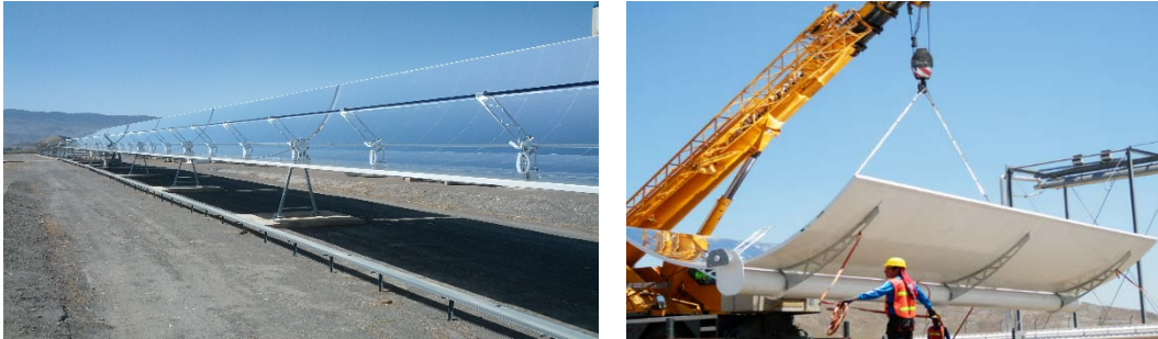
Figure 43. Solarlite DSG Trough (SL 4600) installed in Thailand. Photos from Solarlite, credit: Solarlite.
