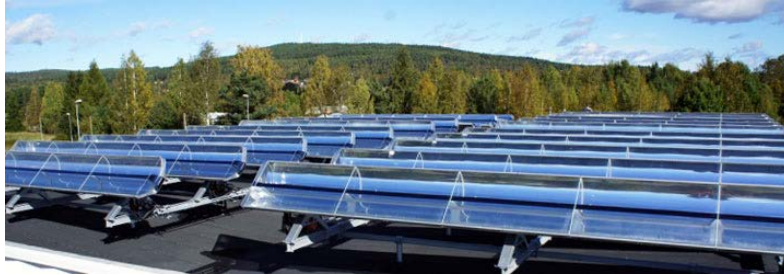
Figure 32. Absolicon T160 roof mounted solar field at the Smedjebacken Industrial park in Sweden (Absolicon 2012). Credit: Absolicon.
