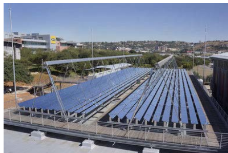
Figure 44. Industrial Solar DSG LF collector roof mounted in South Africa, where the heat is utilized for solar cooling (Industrial Solar 2016)
