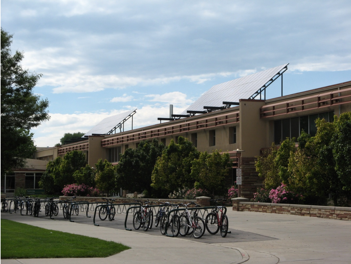
Figure 3. Rooftop PV system on the Engineering Building at CSU's main campus in Fort Collins
