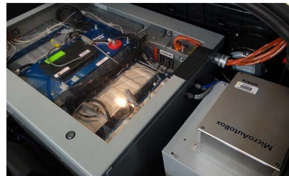
Figure 12. Installed Maxwell EDLC seven-module configuration. Image by Jon Cosgrove, NREL
