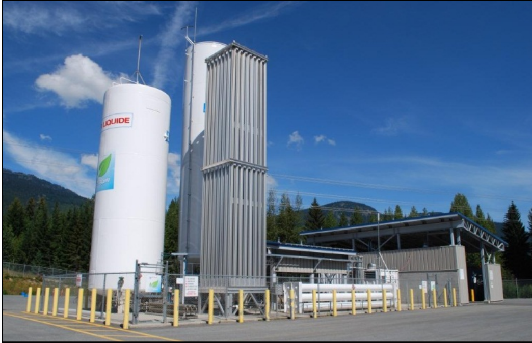
Figure 4. Air Liquide hydrogen station at Whistler Transit Centre
