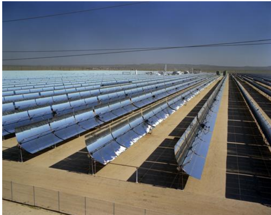
Figure 2-4. Aerial view of CSP trough plants at Kramer Junction, California (in operation for 30 years). Photo by Warren Gretz, NREL 01225
