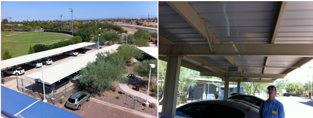
Figure 5-12. Northwest carports looking northwest (left) and carport structure, which would require the attachment of PV support racking (right). Photos by Otto VanGeet, NREL
