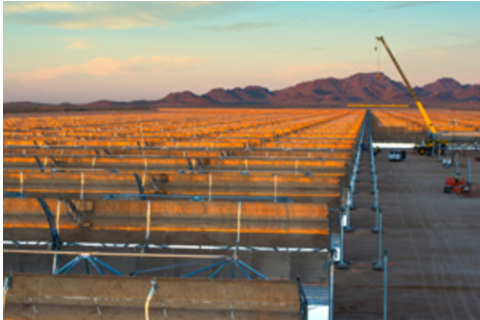
Figure 2-3. 280 MW Arizona trough plant. Photo by Dennis Schroeder, NREL 20097
