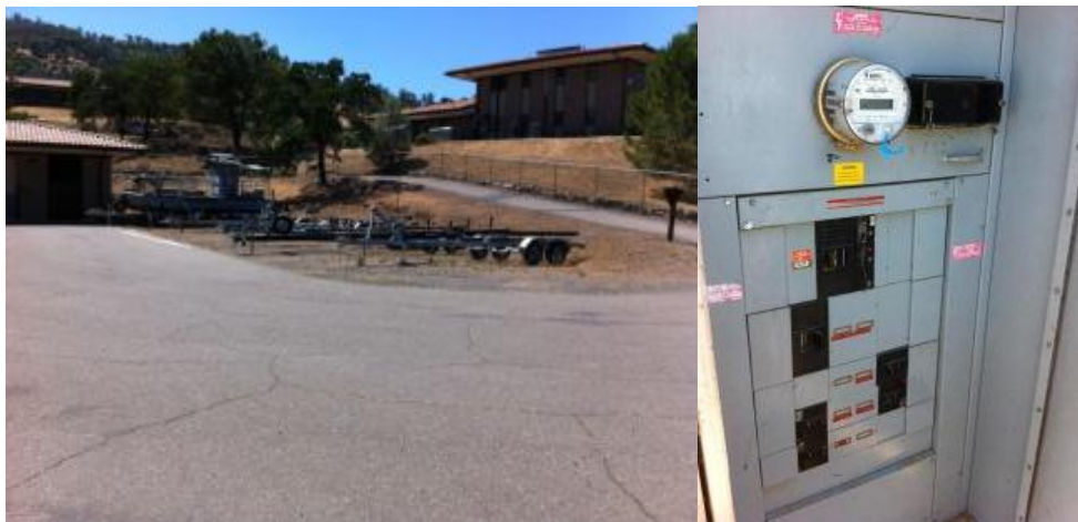
Figure 6-17. PV Carport Area 2: looking northeast (left), and main meter and electrical panel that serves south buildings at Lake Berryessa and possible PV tie in location (right). Photos by Otto VanGeet, NREL
