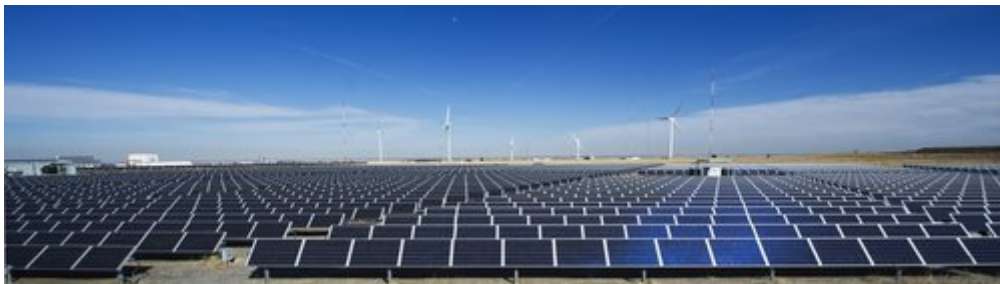
Figure 2-14. Photovoltaic field at the National Wind Technology Center. Photo by Dennis Schroeder, NREL 19794
