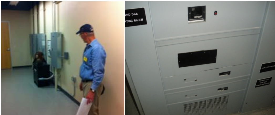
Figure 5-10. Panel LP2A is located in the electrical room near the roof. Photos by Otto VanGeet, NREL
