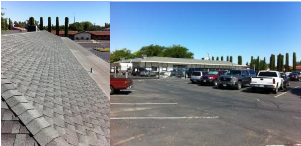
Figure 6-7. East roof of Willow building looking north (Area 1) (left), and east side of building and roof looking northwest (right). Photos by Otto VanGeet, NREL
