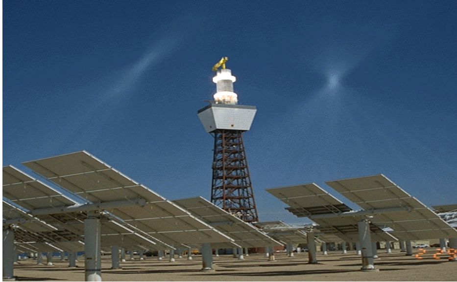
Figure 2-6. DOE solar demonstration power tower in southern Nevada. Photo from Sandia National Laboratories, NREL 06051
