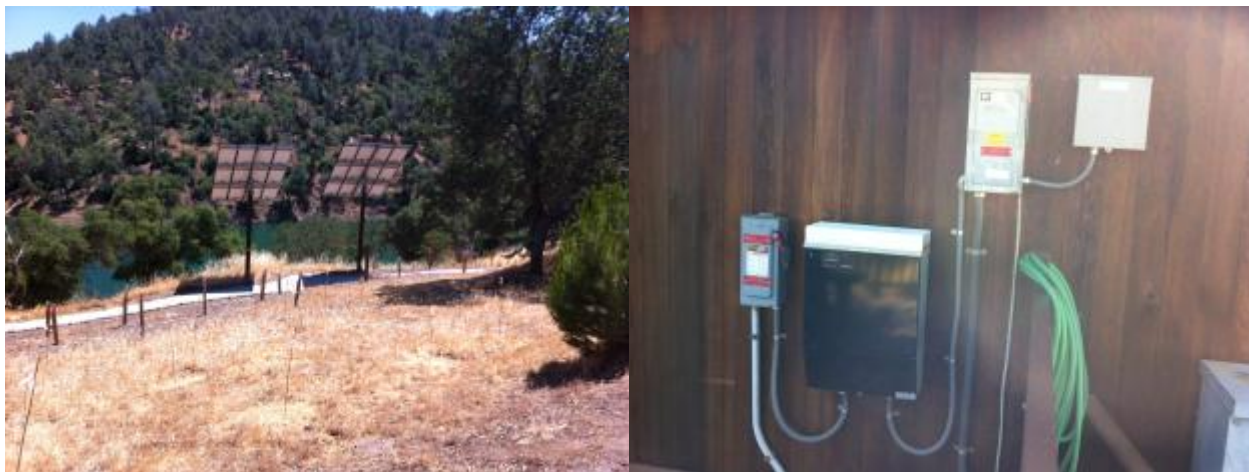
Figure 6-11. Existing PV system and inverters at Lake Berryessa Office (existing PV 1). Photos by Otto VanGeet, NREL
