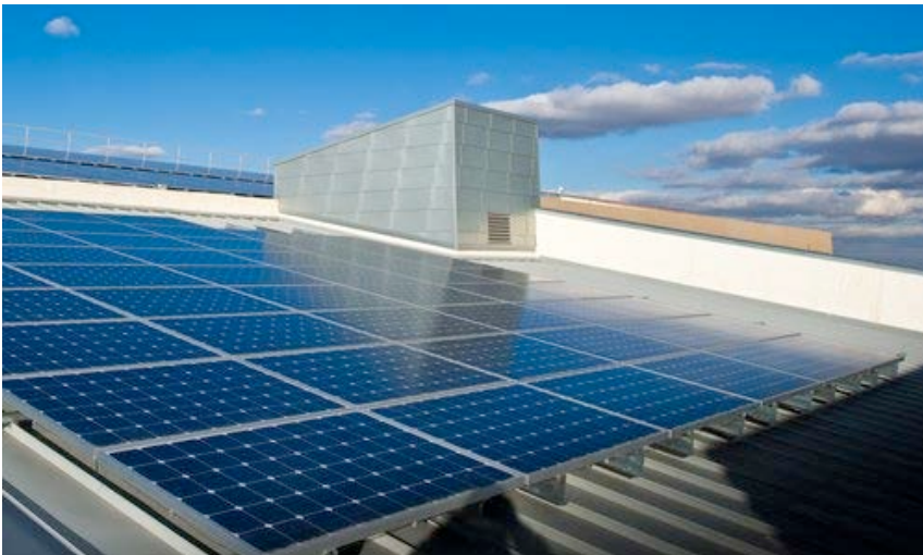
Photo by Dennis Schroeder, NREL/PIX 19547
