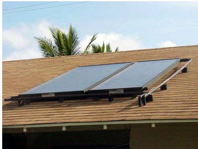
Figure 20. Residential Solar Hot Water, Hickam AFB, Hawaii
