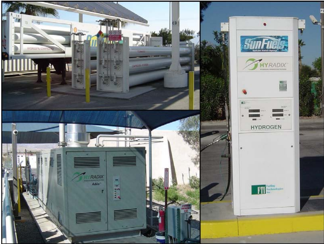
Figure D-6. SunLine's hydrogen storage (top left), HyRadix Adéo commercial reformer (bottom left), and hydrogen dispenser (right)
