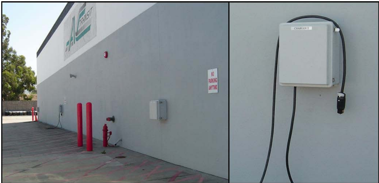
Figure D-7. Fuel cell bus/battery charging station at AC Transit
