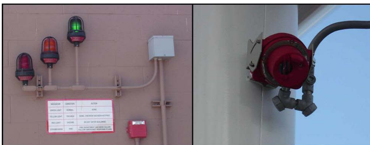
Figure D-5. Condition indicator lights (left) and hydrogen flame sensor (right) at the Chevron—AC Transit Hydrogen Energy Station
