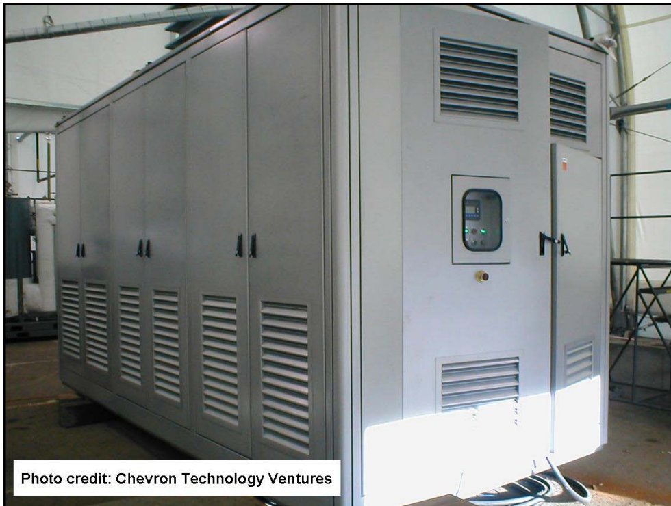
Figure D-2 Primary reformer at Chevron—AC Transit Hydrogen Energy Station (75 kg/day)
