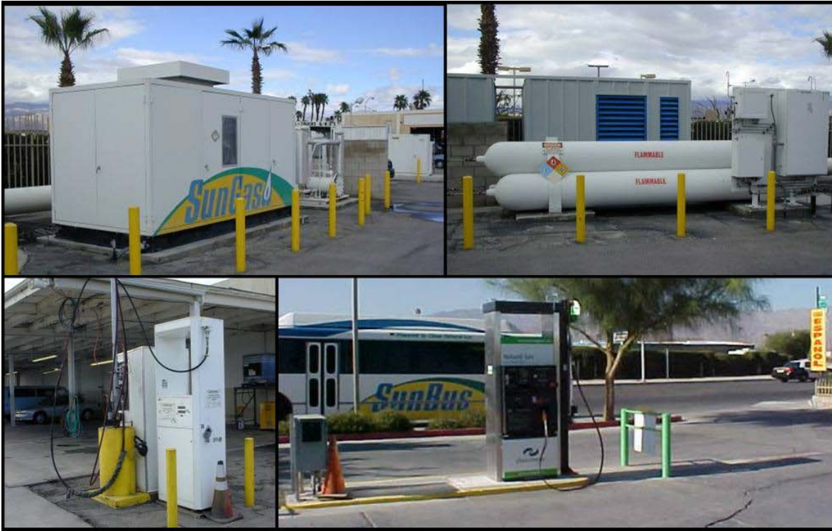
Figure C-4. CNG fueling equipment (Indio)
