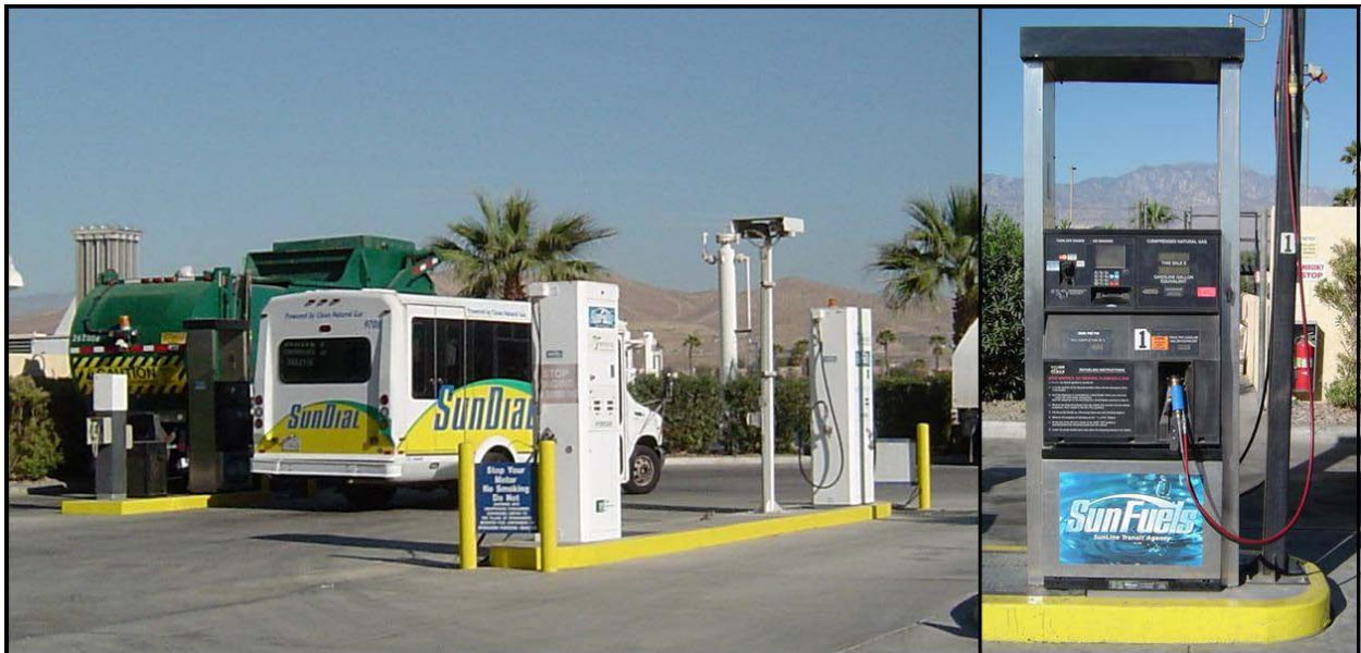
Figure C-1. Public fueling at SunLine's Thousand Palms CNG fueling station
