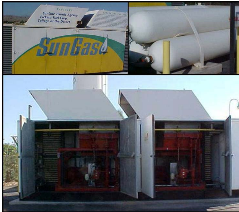
Figure C-3. CNG compressor station (Thousand Palms)
