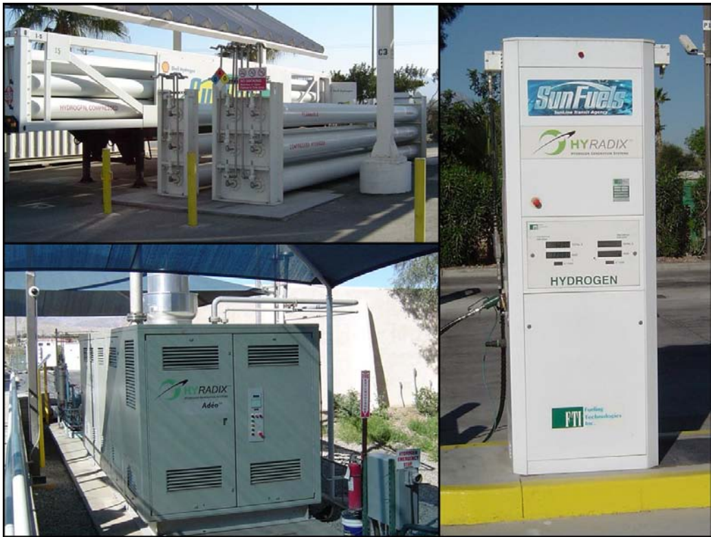
Figure C-6. SunLine's hydrogen storage (top left), HyRadix Adéo commercial reformer (bottom left), and hydrogen dispenser (right)
