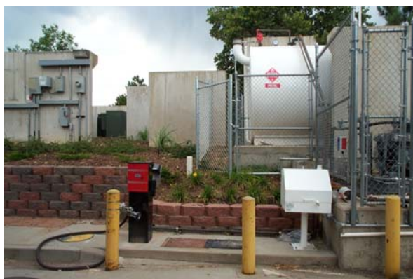
Figure 2. B20 Fueling Station
