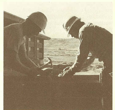
Laboratory facilities were under construction the first year for completion in early 1979.
