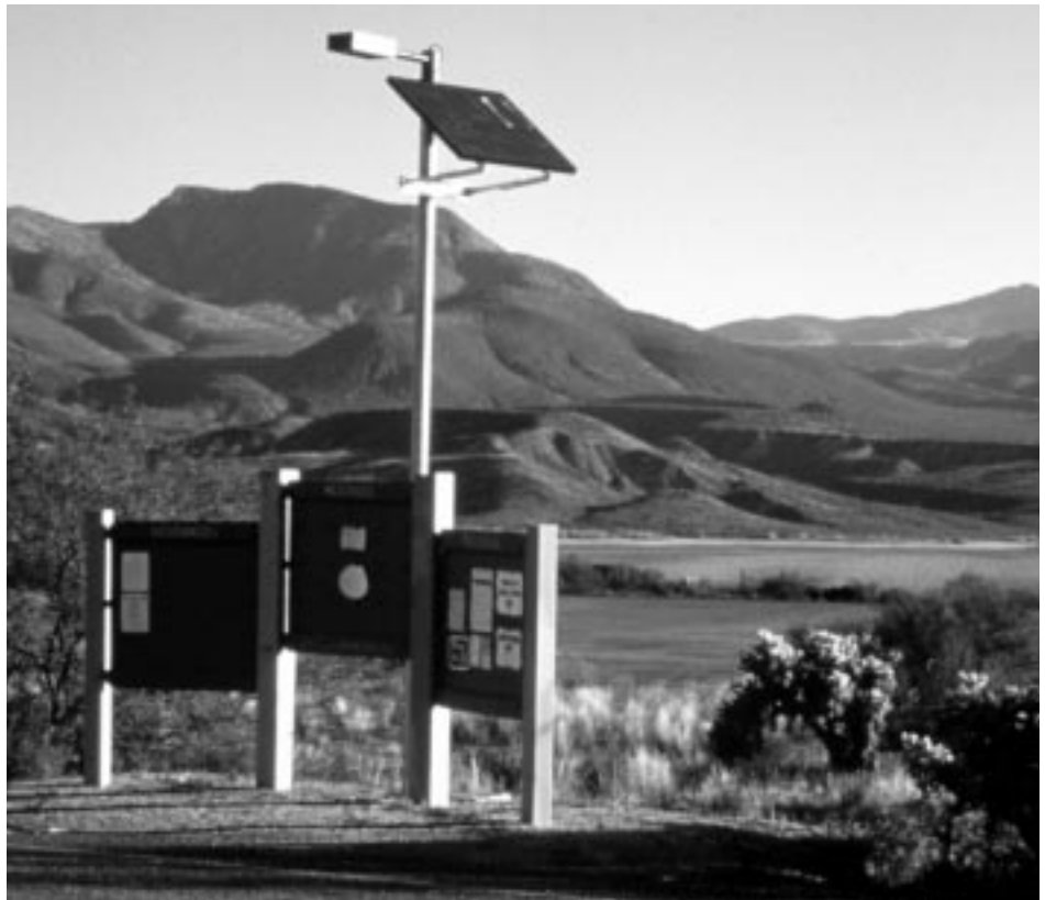
Figure 1. PV lighting system at Roosevelt Lake in Phoenix, Arizona.
