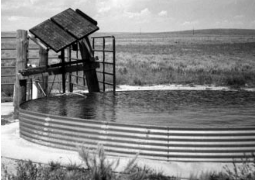
PV-powered water pumping on a Colorado ranch.
