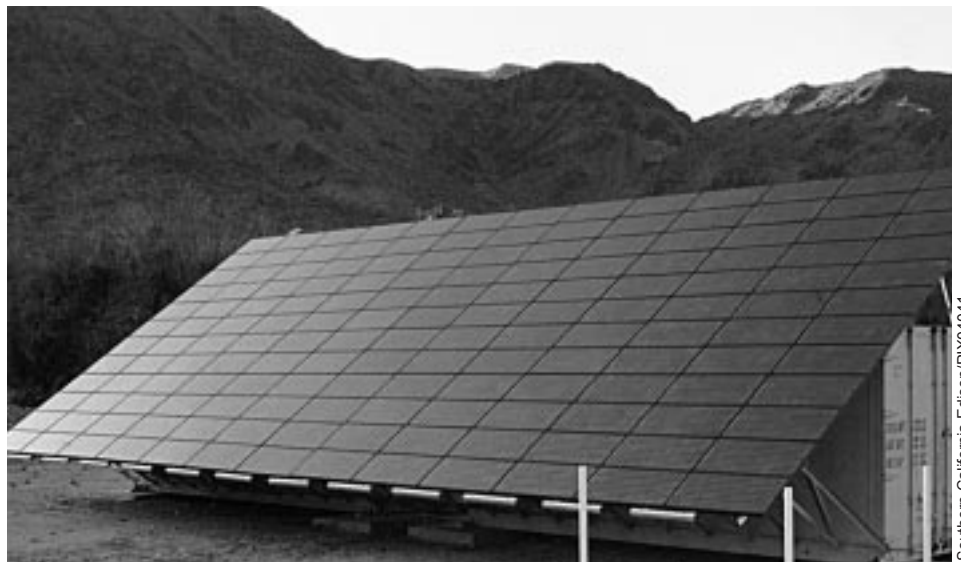
A portable PV/propane hybrid system provides electricity for the California State University Desert Research Center in Southern California.
