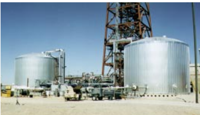
Storage is the key to molten-salt power towers. These two tanks provide three full hours of storage at Solar Two.
