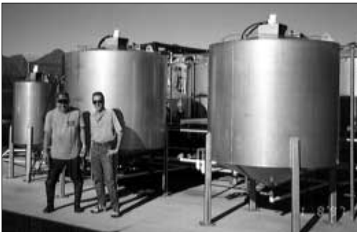
Larry Zolezzi and Carl Nagata at Pacific Biodiesel plant in Maui
