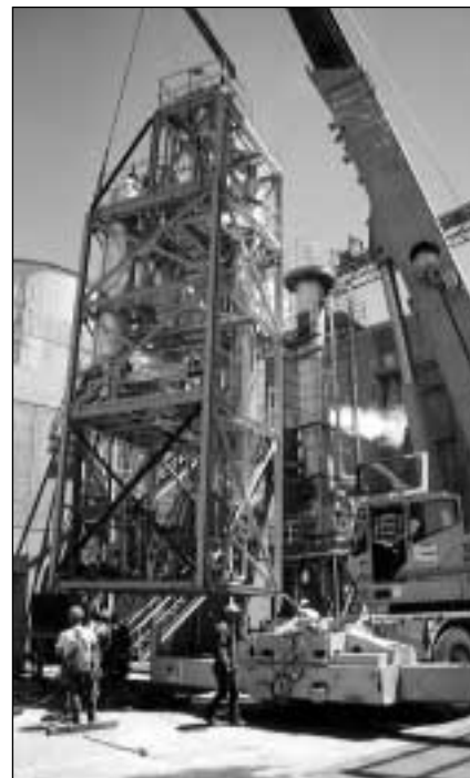
This mole sieve dehydration unit is part of the plant within Coors Brewery that recycles waste alcohol condensate and produces ethanol.
