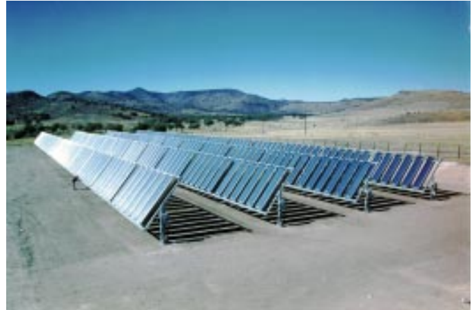
100-kW system at CSW Solar Park in Ft. Davis, Texas.
