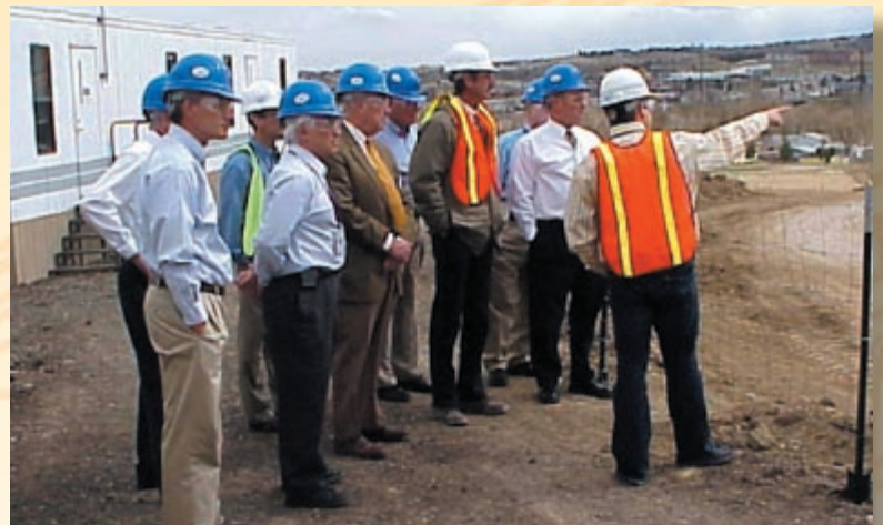
MRI Board Oversight Committee completed an external independent review of S&TF construction with no findings or concerns. The S&TF is on track to receive a LEED Gold rating.
