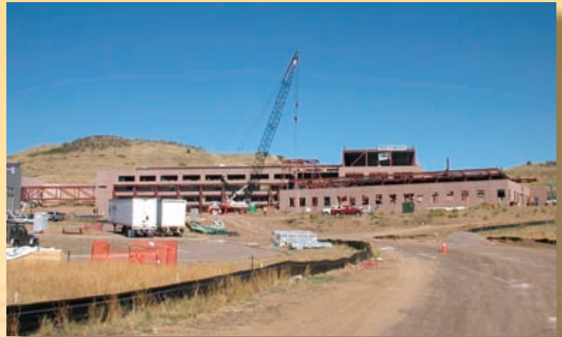
The S&TF construction is on schedule and interior work is proceeding. The facility is expected to be ready for occupancy in mid-2006.
