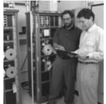
Located at the Solar Energy Research Facility, these control panels monitor the potential release of toxic gases.
