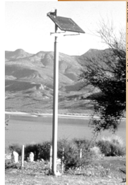
PV-powered security lighting at Roosevelt Lake in Arizona.
