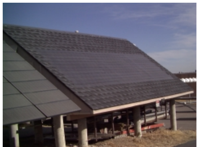
Figure 1. Roofing Shingle PV System
