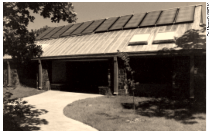
Visitors now enjoy hot showers at Chickasaw National Recreation Area, thanks to solar water heating systems such as the one installed on this large comfort station.
