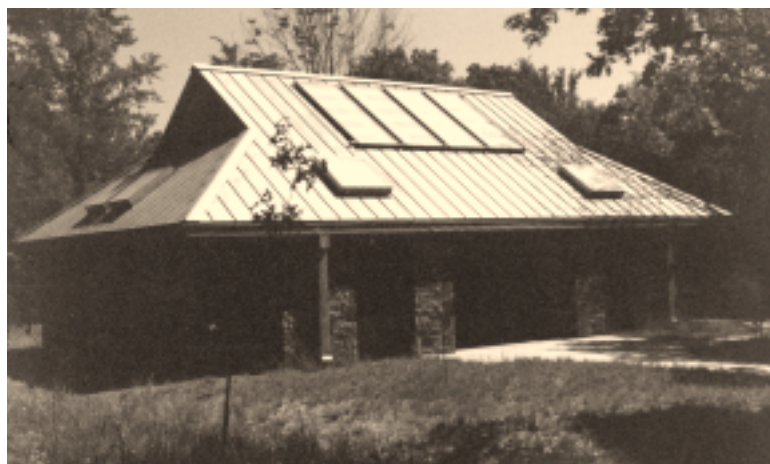
The solar hot water system on this small comfort station at Chickasaw National Recreation Area supplies all the hot water for the building. There is no backup system.
