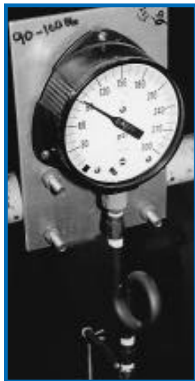
Figure 3. Elevated pressure gauge with loop seal.
