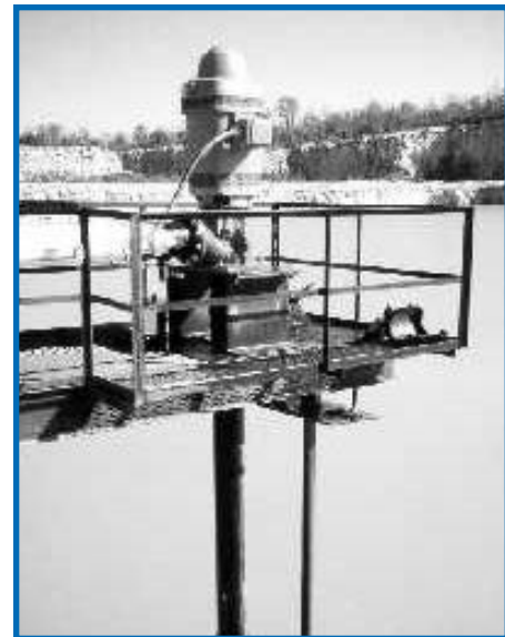
Water pump at Blue Circle Aggregates' Lithonia quarry.
