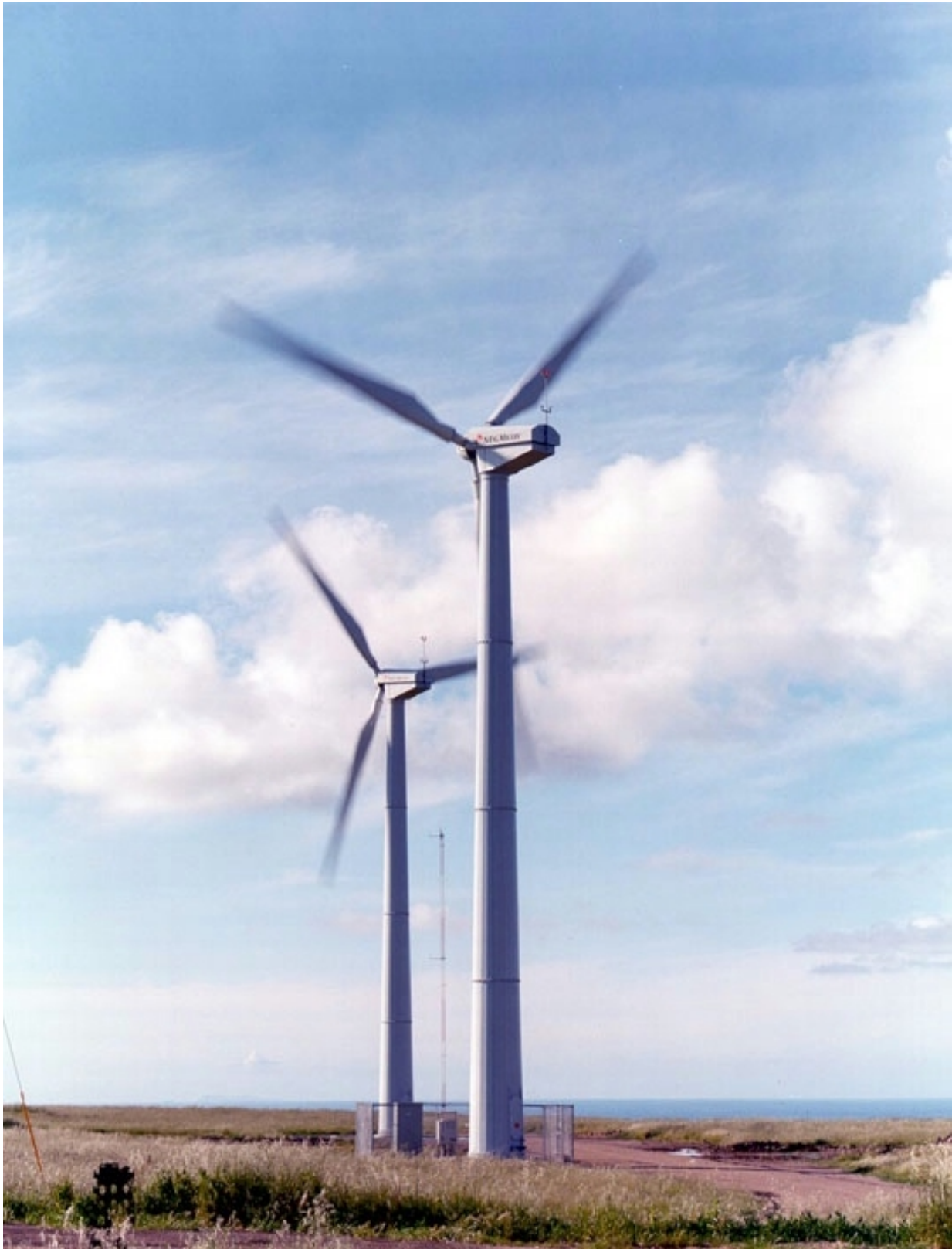
Figure 10: SCI SERDP-Funded NM 225-30 (225 kW) Wind Turbines Source: USN NFESC Photograph
