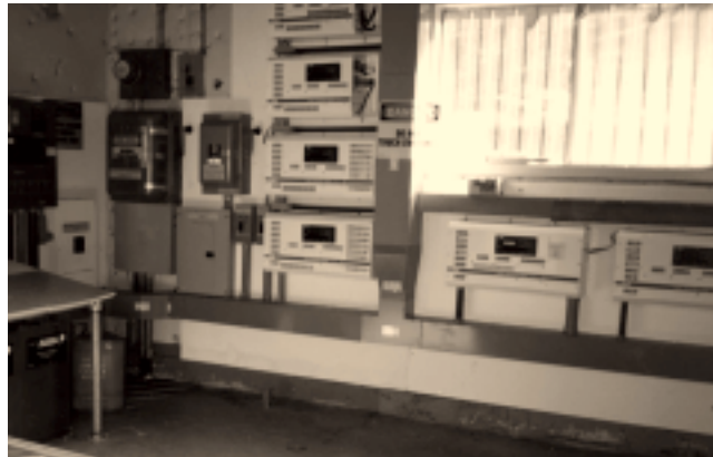
The designers divided the electrical service into two separate single-phase lines to keep the maximum single-phase load below 16 kW, which allowed the use of less expensive off-the-shelf inverters. All the equipment for this project was purchased off the General Services Administration supply schedule.
