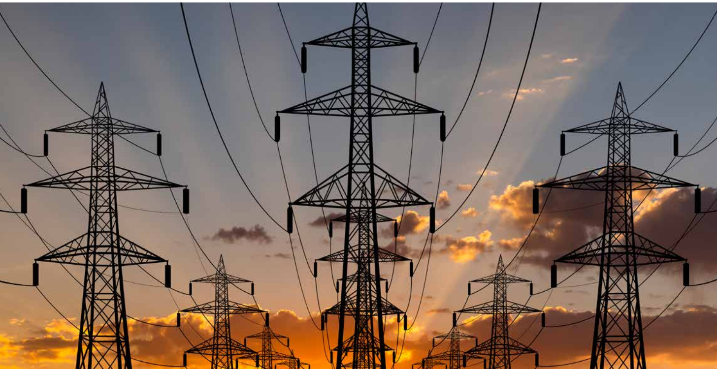
NREL researchers partnered with Xcel Energy to use NREL's EVI-DiST to provide standards development guidance on infrastructure upgrades to prepare for growing EV charging loads.
