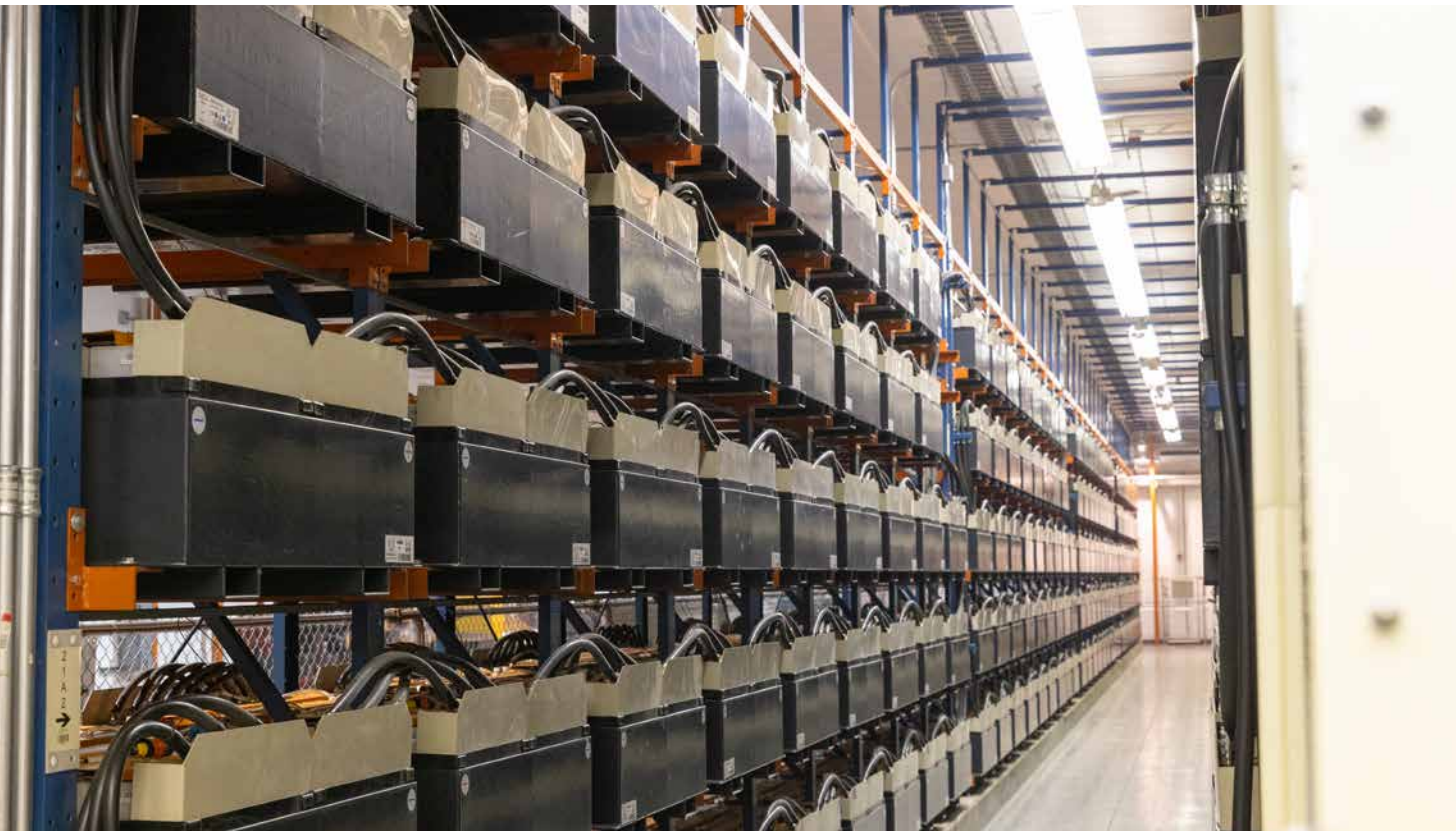
Inside the battery energy storage system at the Golden Valley Electric Association's (GVEA's) facility in Fairbanks, Alaska. Behind-the-Meter-Storage systems such as this one can help manage demand charges, provide continuous energy supply during power outages, enable EV fast charging, and more.
