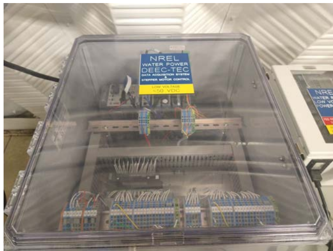
Fig. 3. Electronics enclosure with the cRIO and modules in the back, the PLC511 motor controller in the middle, and wire connections in the front.
