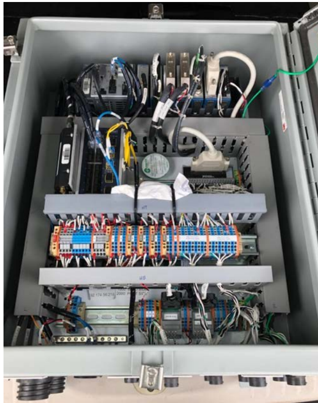
Figure 4. A MODAQ system is packaged in a stainless-steel enclosure for field deployment.
