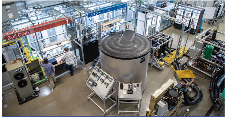
Figure 2. Commercial buildings labs emulate the grid and environment with real building equipment and the ability to switch to any building or location.
