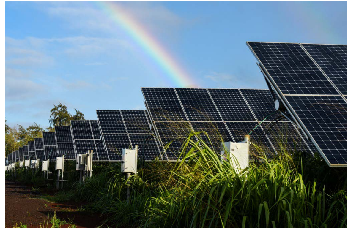
Photo by Dennis Schroeder, NREL
