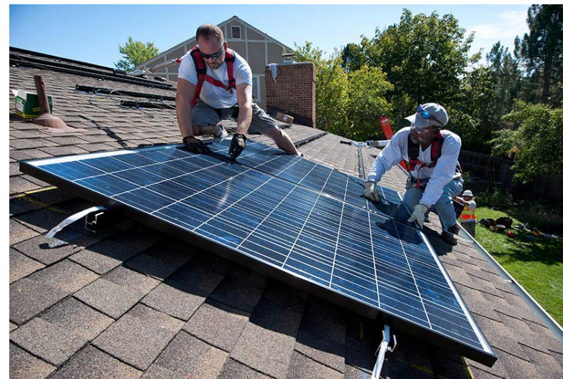
Photo by Dennis Schroeder, NREL
