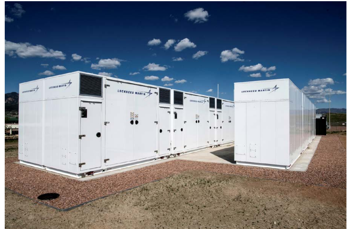
Utility-scale lithium-ion battery energy storage system installation. NREL Image 31411.
