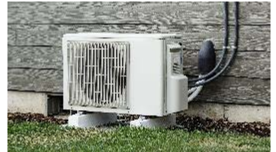
Ductless heat pump outside compressor. Image from Building America Solution Center
