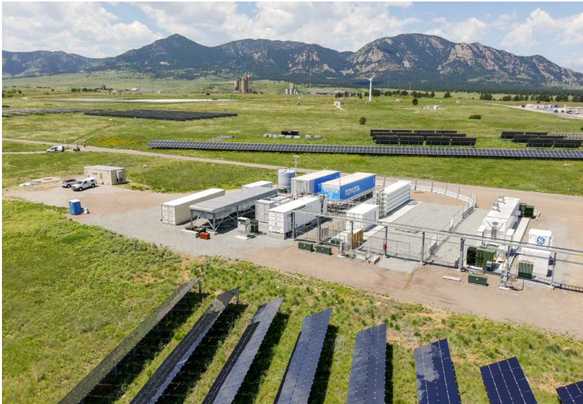
Aerial view of the hydrogen infrastructure and grid integration research pads at National Renewable Energy Laboratory's (NREL's) Flatirons Campus. These capabilities are part of the ARIES research platform. Photo by Josh Bauer/Bryan Bechtold, NREL 82063
