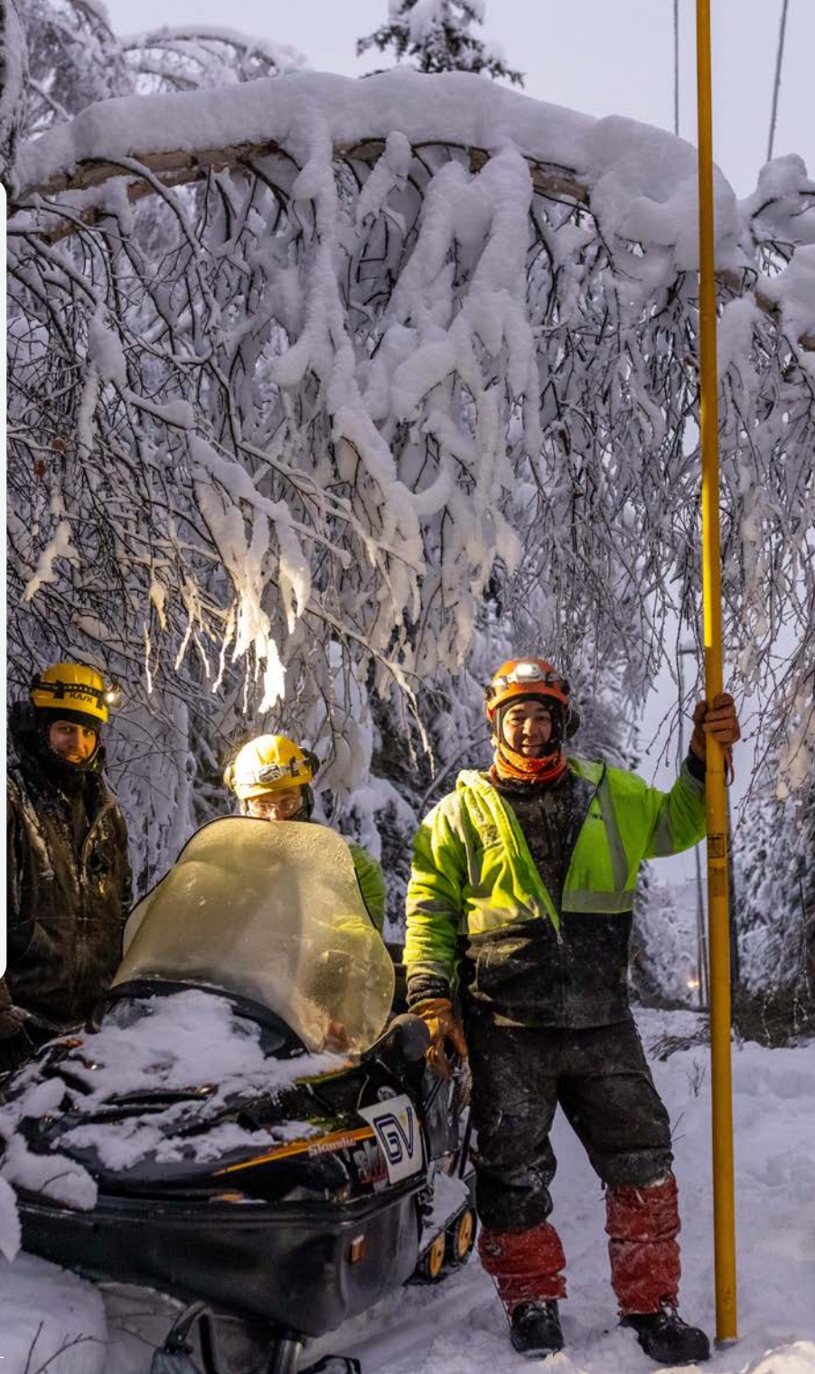
Photo from Golden Valley Electric Association, Fairbanks, Alaska
