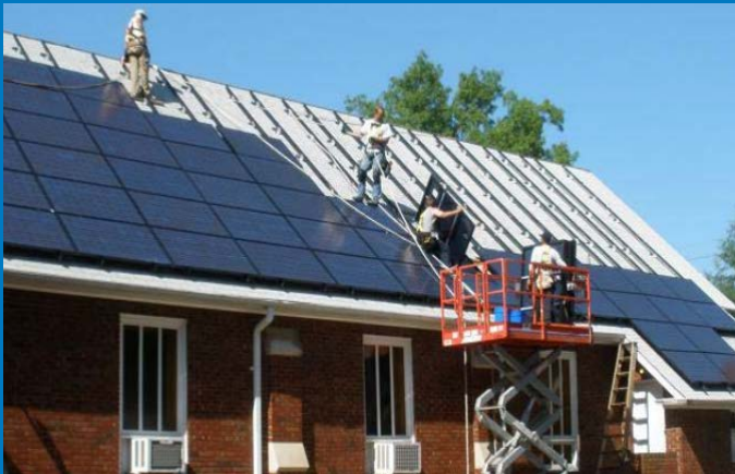
Source: Photo from David Brasch, University Park Community Solar, LLC
