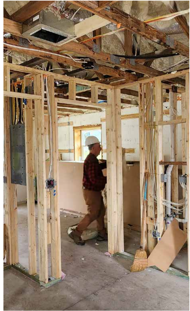
Characteristic wall and ceiling layout for 1/1 design. Photo by Jeremy Gary, Building Performance Consultants Inc.
