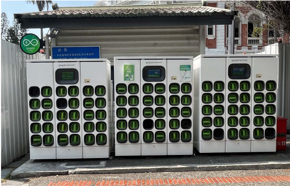
Figure 5. Gogoro battery swap station in Taiwan.
