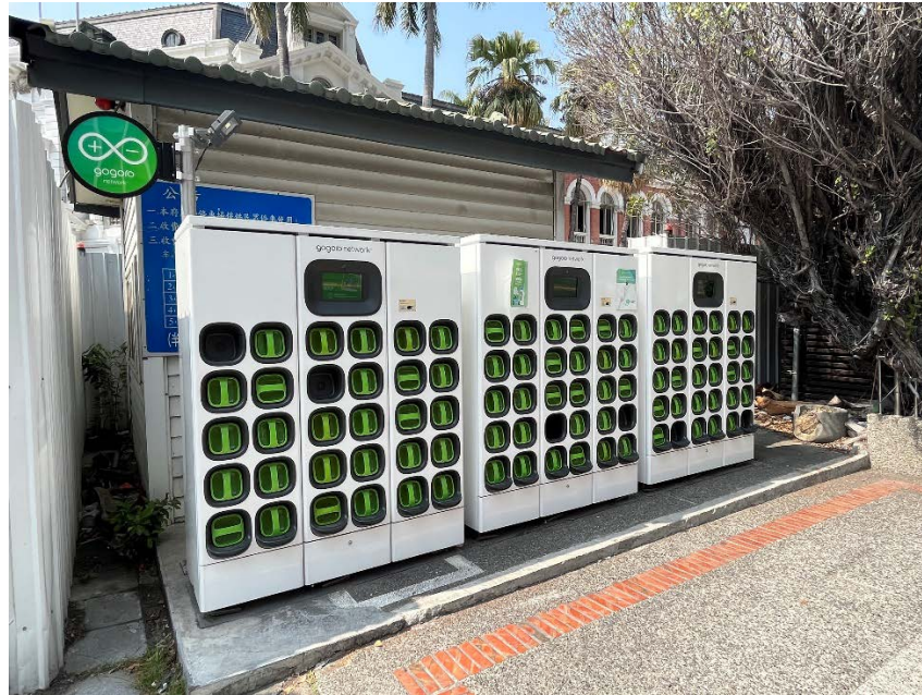
Figure 17. Gogoro battery swap station in Taichung City, Taiwan.
