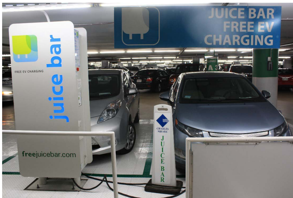
Figure 22. An EV charger sign in the United States advertising free charging.
