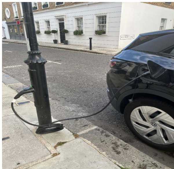
Figure 13. Mode 3 charging station built into a streetlight post with an untethered cable.
