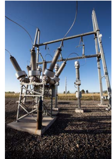
Photo by Dennis Schroeder, NREL 62223
