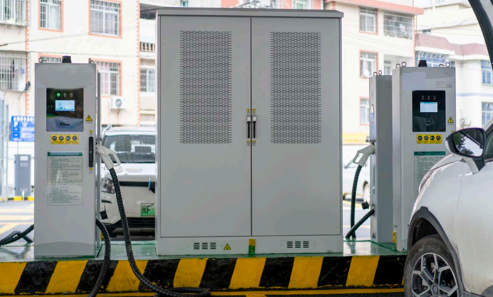
Demand for transformers for EV charging stations is set to increase. Photo from Getty Images 1421282386
