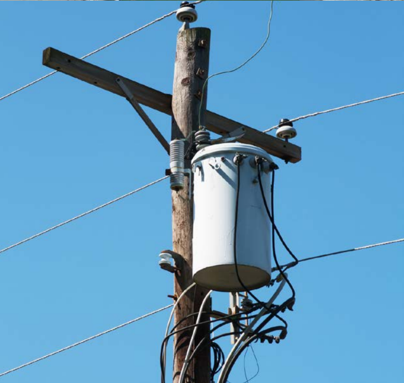
While pole-mount transformers account for the most orders of transformers by numbers [23], pad-mount demand is expected to increase as utility investment in undergrounding and resilience programs increases. Photos from Getty Images, top: 1388647482, bottom: 152264156
