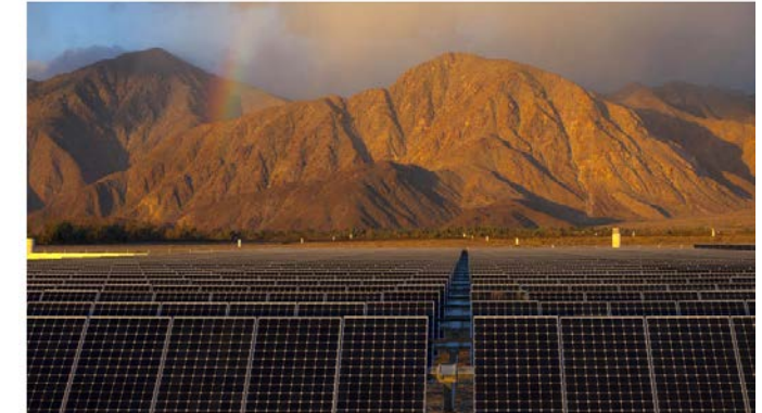
San Diego Gas and Electric (SDG&E) considers this to be the first utility-owned, community scale microgrid in the country. Photo by SDG&E [10]
