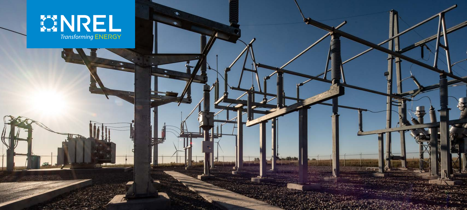
Photo by Dennis Schroeder, NREL 62227
