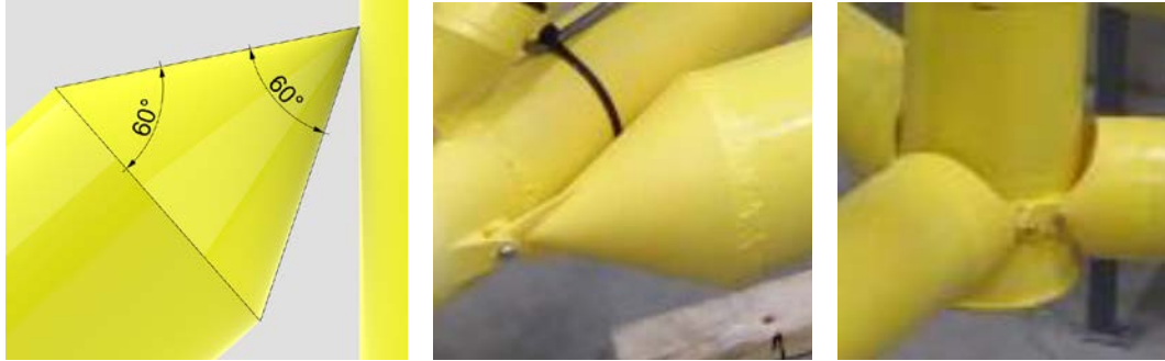
Figure 19. Node connections: left - modeled characteristic node cross section, center – experiment characteristic node (Allen and Fowler 2019), right – central column connection (Allen and Fowler 2019)
