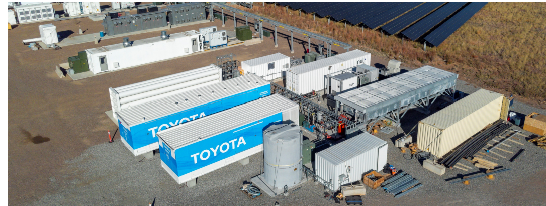
Installed hydrogen system at NREL's Flat Irons Campus. Photo by Josh Bauer/Bryan Bechtold, NREL 73051
