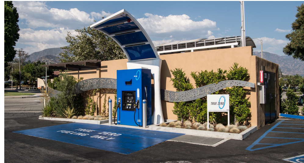
Figure 6: Light-duty H 2 fueling facility in La Cañada, CA.
