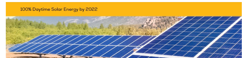
Kit Carson Electric Coop (KCEC) solar panels generate daytime power. Photo by KCEC https://kitcarson.com/electric/100-daytime-solar-energy-by-2022/ .
