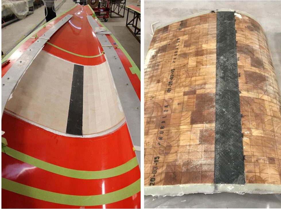
Figure 6. End grain balsa blocks attached to a scrim backing within a blade mold (left) and post infusion (right). Photos by Ryan Beach, NREL
