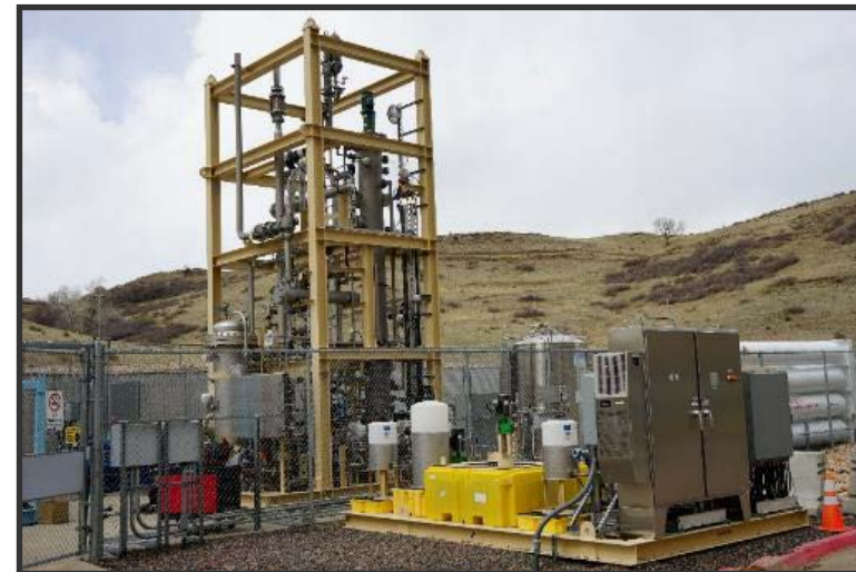
Biomethanation reactor (NREL)
